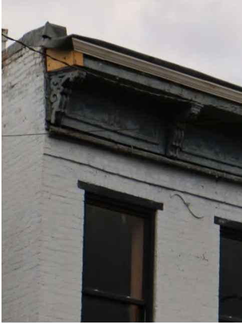
REPAIR NOT COVER. Deteriorated sections of cornices are to be repaired in-kind or with compatible materials. Long-term or permanent covering over of deteriorated cornices is not an appropriate alternative to repair.
